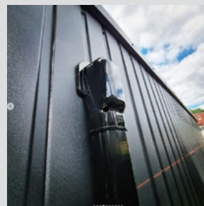
Photo provided by JMG Cooling Services (UK)
